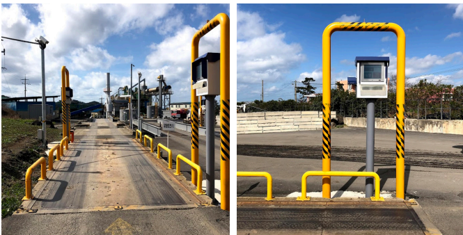
Weighbridge and automatic measuring equipment installed at the entrance of a waste disposal facility
