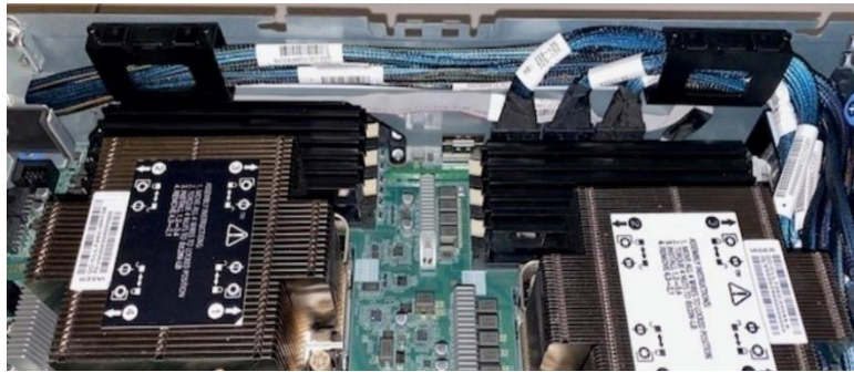
Figure 17. Internal Cable Management
