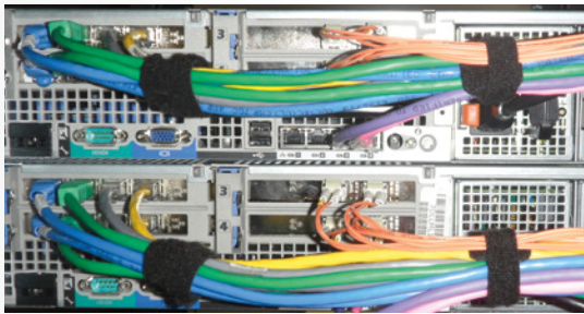
GbE Server Connections
