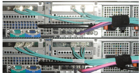
10 GbE Server Connections
